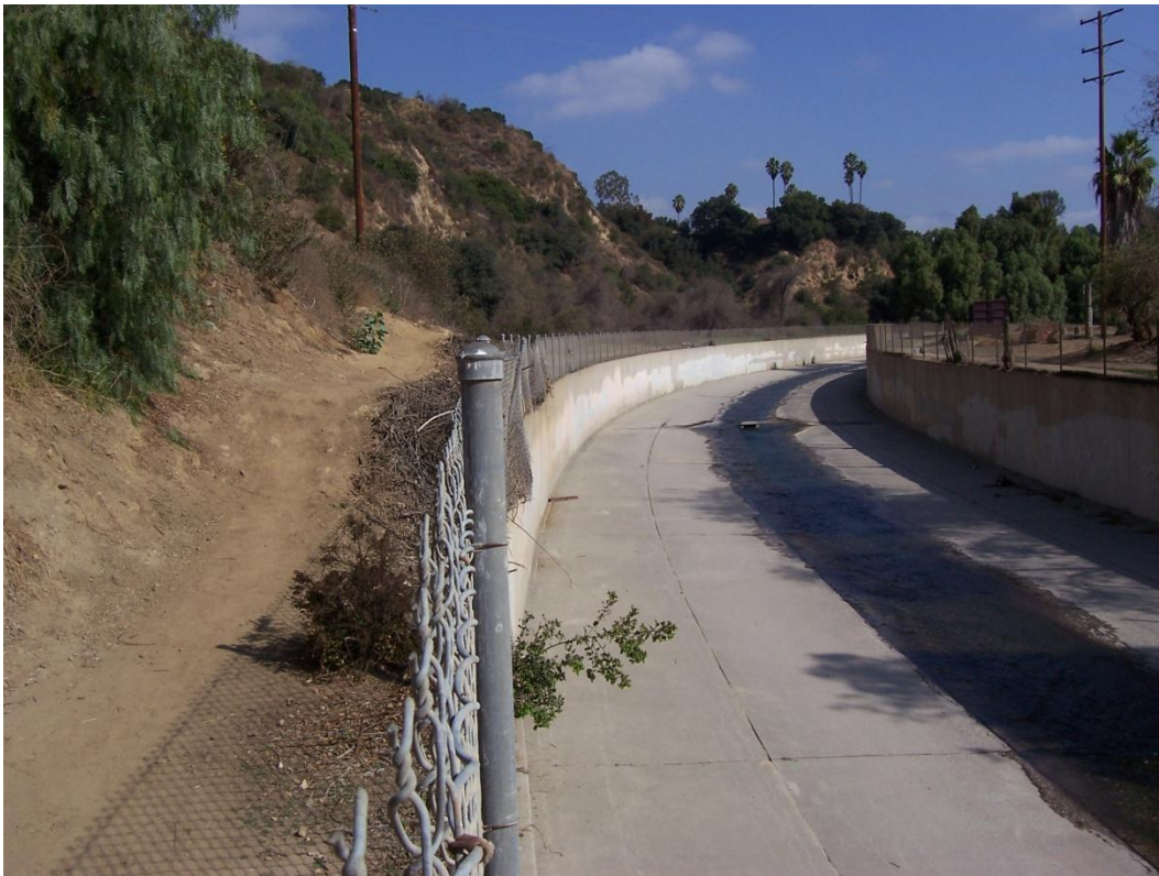
Section 2509 Looking Upstream Right Bank Mudslide
